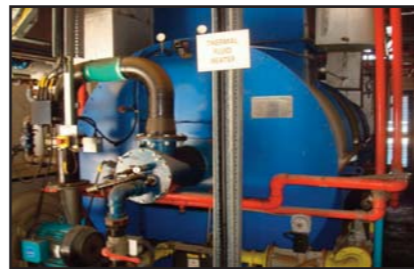
STOCK CODE: NS0018-22 1600KW CONTRAPOL THERMAL FLUID HTR
