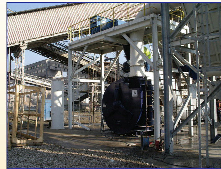
Pulverised fuel production in Poland
